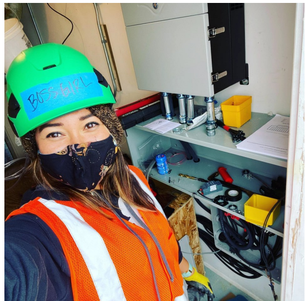
Deilah Johnson during July 2021 solar install at community center, pictured as a selfie when the first combine box attached to the inverter was just placed in the former tool shed.
